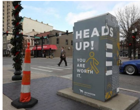
An example of a signal cabinet box promoting pedestrian and bicyclist safety in Lexington, Kentucky. (Source: Lexington Herald Leader)
