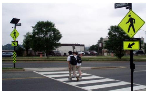
Rectangular Rapid-Flashing Beacon (RRFB)
